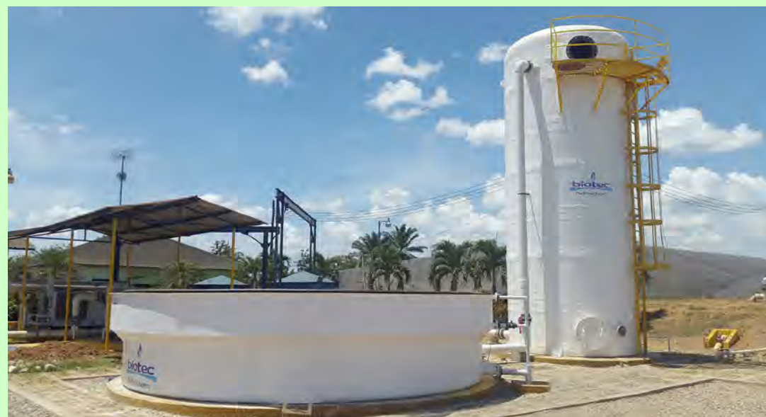
AGUAN, Biogas Plant
